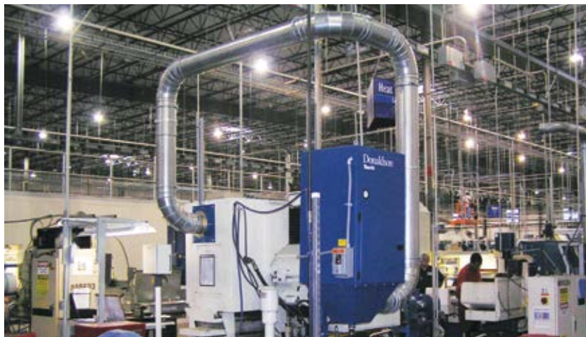
WSO - Machining Center 1,200 cfm (2,038m 3 /h)
